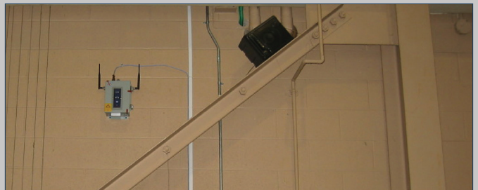
Secure wireless in hangar
