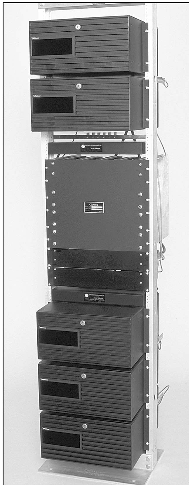
Figure 2-4 Rack Mounted Repeaters
